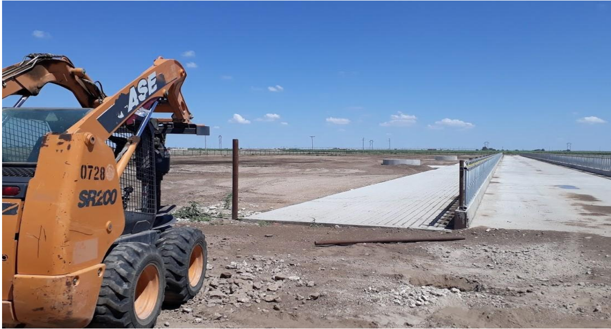
Figure J: Cheap new US milk. Expanding mega farm in New Mexico: strip of concrete, water trough and wire fence around dirt pens.
