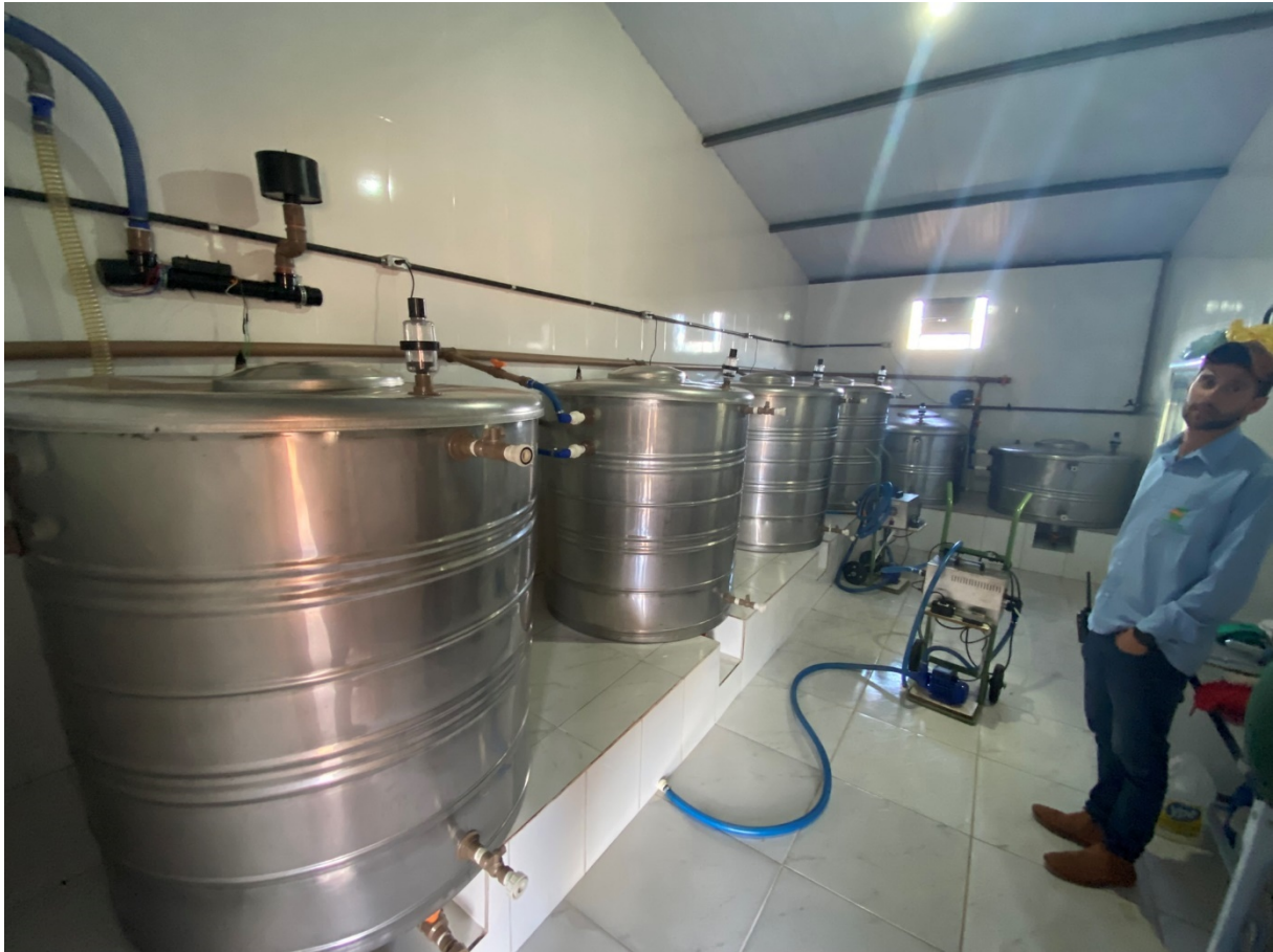
Figure 4: Installation for the multiplication of microbiological preparations, Brasil. (Source: Author)
