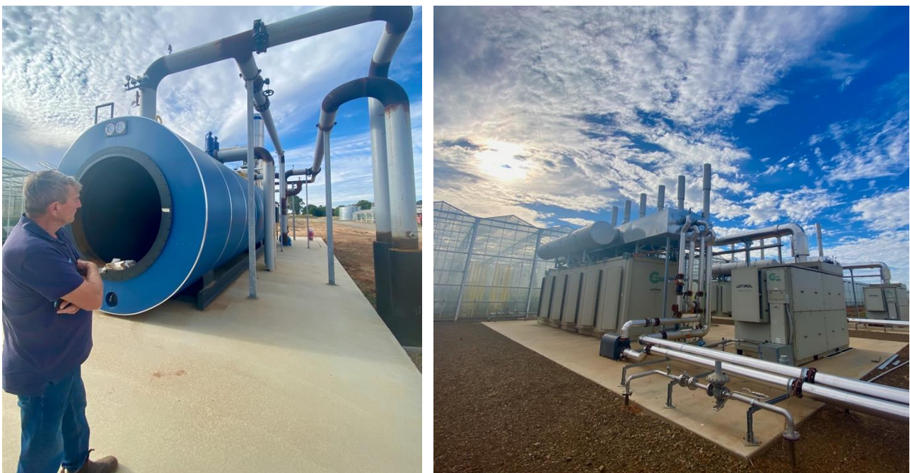
Figure 15: The boiler (left) at Katunga Fresh in Victoria, Australia, heats the glasshouses during the winter, and the ORC generators (right) produce electricity during the summer. Both will be fuelled from the excess gas of the pyrolysis system. (Author's own)
