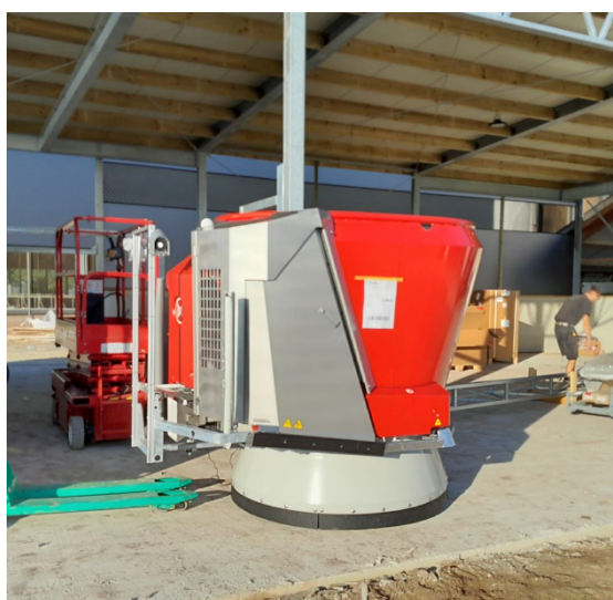
Figure 3: The new Lely automated feed system being installed on the Elferink family farm, Netherlands.
